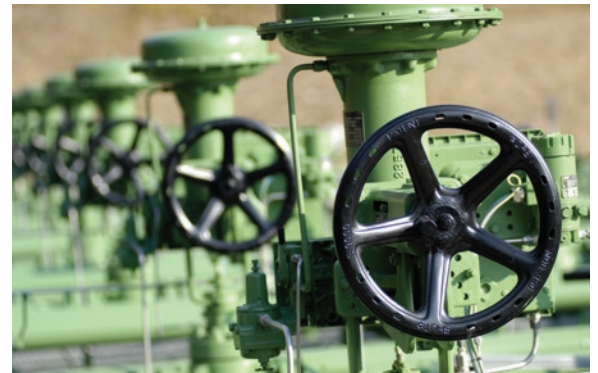
Detail of gate valves. Gas storage facility in Collalto (Treviso).
