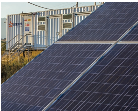
Edison field in Altomonte: solar panels with storage battery
